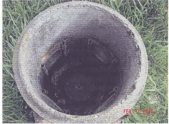
Photograph 14: Stand pipe on Parcel 1 adjacent to fence. Liquid and solid at base.
