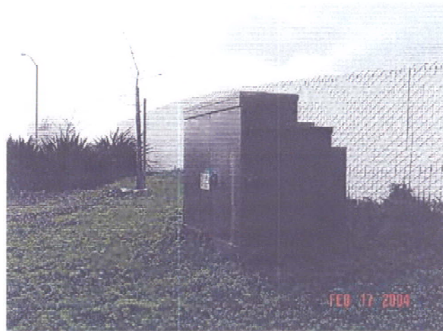
Photograph 9: Pad mounted transformer onsite not labeled as to PCB content.
